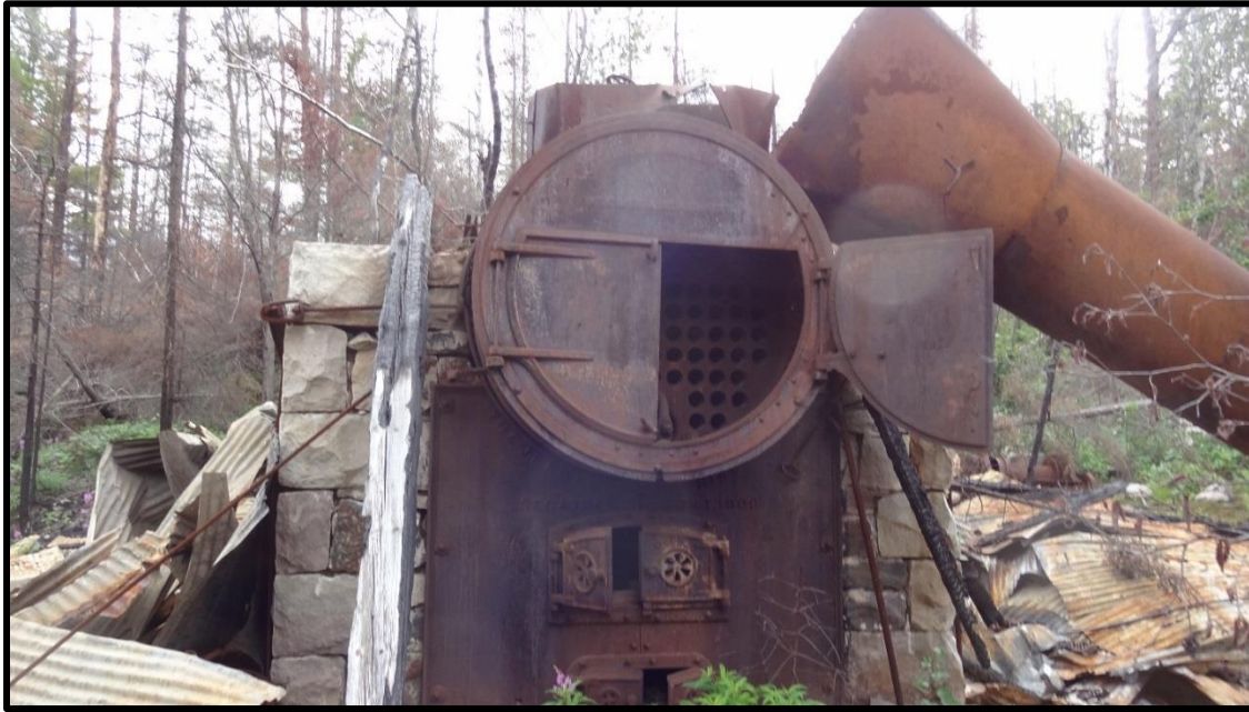
Photo 1: 1909 Minesite boiler after the 2018 forest fire
