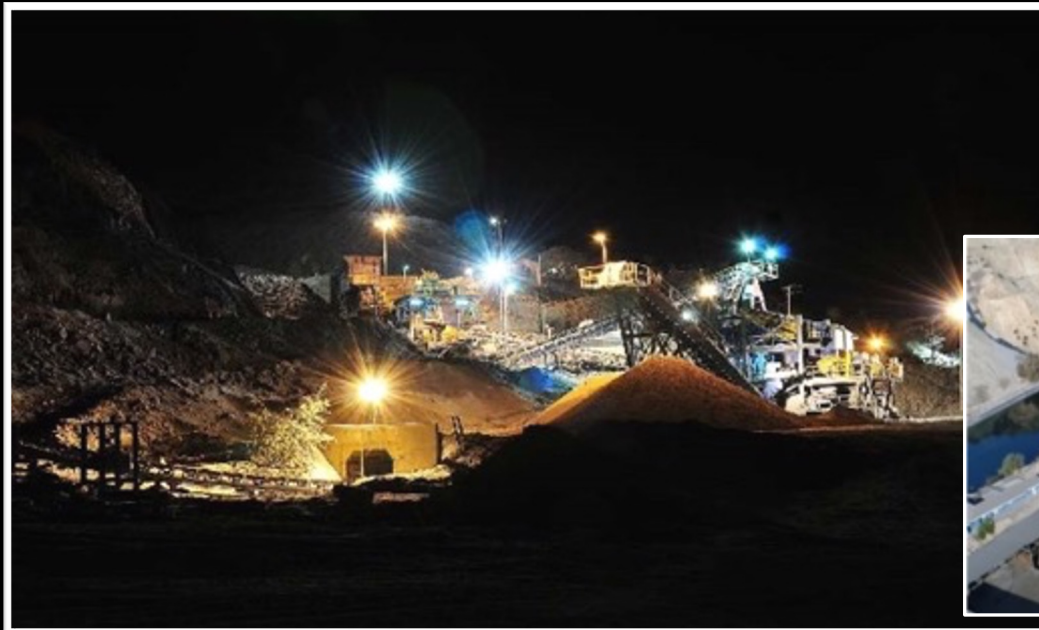
View of the Punitaqui plant operating at night (Feb 2020)
