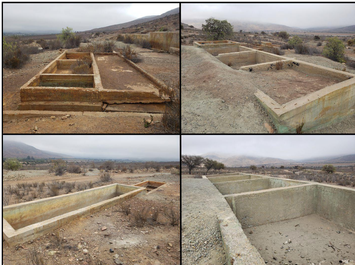
Figure 9-11: Santa Elvira 1980's Vintage Copper Oxide Leach Processing Plant Concrete Footings and Pads
